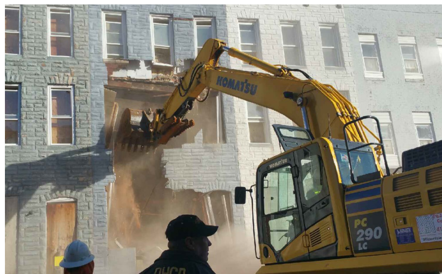
The state's demolition of dilapidated and vacant houses in the Sandtown Winchester area began Jan. 5 with the Governor and Baltimore City Mayor's announcement of the revitalization initiative, Creating Opportunities for Renewal and Enterprise (CORE) on Jan. 5.
